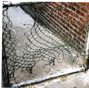
mangled chain-link fence
