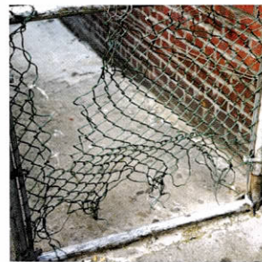
mangled chain-link fence
